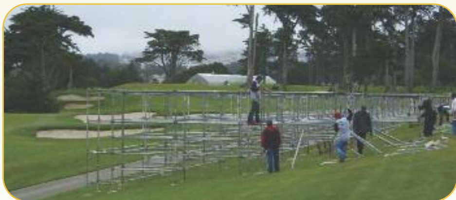
Crew members at Harding Park begin installing bleachers along the golf course
